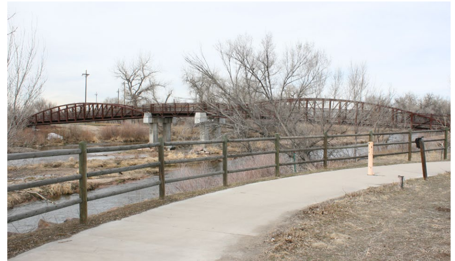
Looking northwest at pedestrian bridge over South Platter River in Fort Lupton
